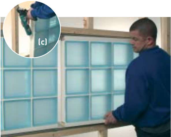
Step 3 : Apply silicone to the connecting joint on the second panel (c). Carefully lift second panel in vertical motion onto plastic packers and slide up to first panel ensuring a neat joint at intersecting point. Note : Apply more silicone if required.
