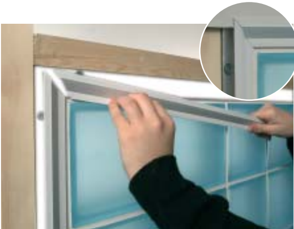
Step 5 : If using plasterboard coverstrip carefully measure, mitre corners and slot into position.
